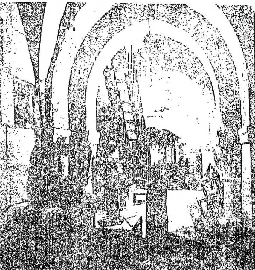
Restoring ornamental bands and columnheads in first floor gallery, which belongs to the Greek Orthodox. Note plaster model of column-head on floor at right.
